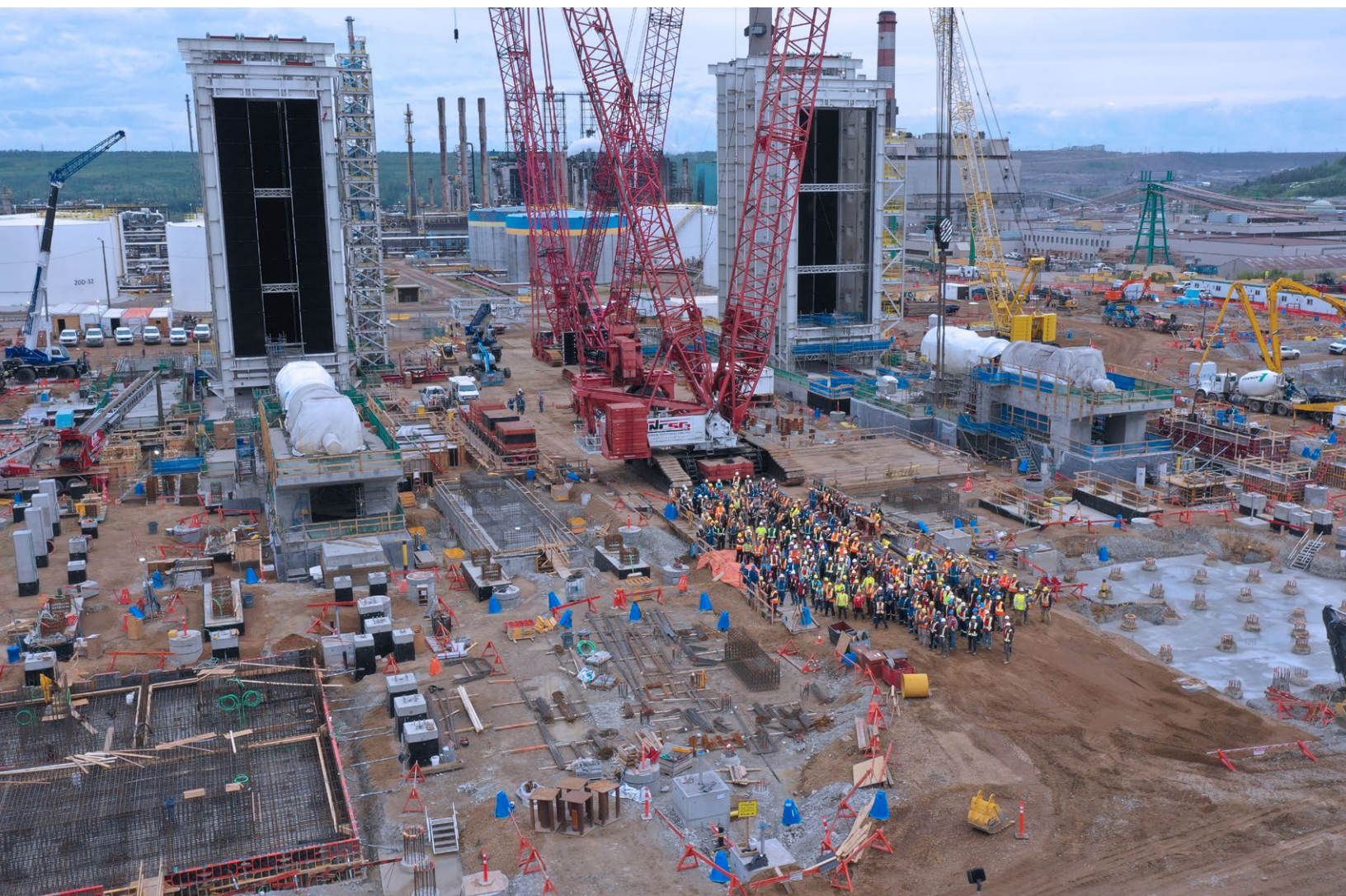
The Base Plant Cogeneration construction team celebrating the setting of the gas turbines and generators.
