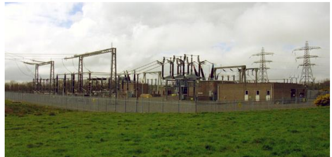
Alverdiscott National Grid substation
